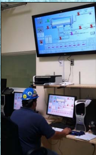
Jim Fritz monitors one of the new plant's first backwash cycles.
